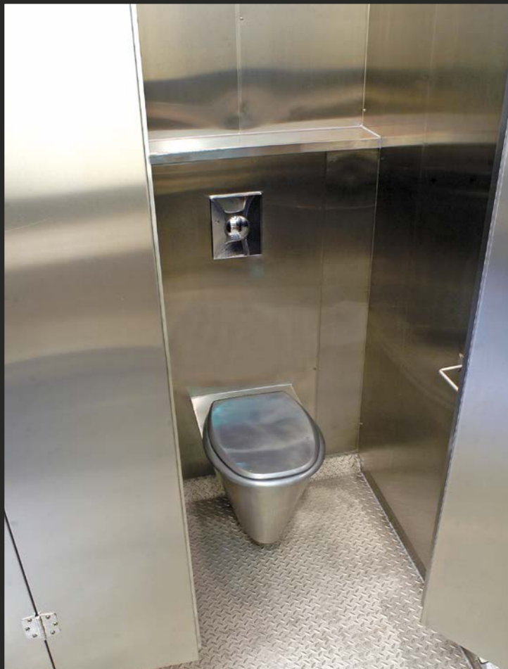
Sanitation container, configured with 3 toilets and 3 showers
