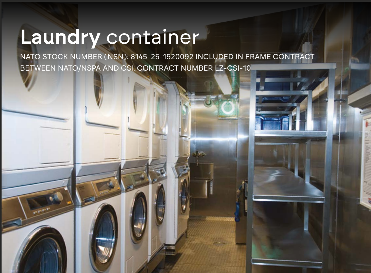
Laundry container with 6 Miele industrial washing machines and 6 industrial tumble dryers
